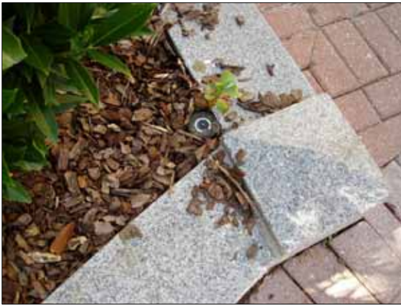
Irrigation heads are protected by curbing.
